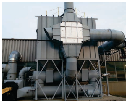
Ship & Shore RTO with Heat Exchanger for waste heat recovery
